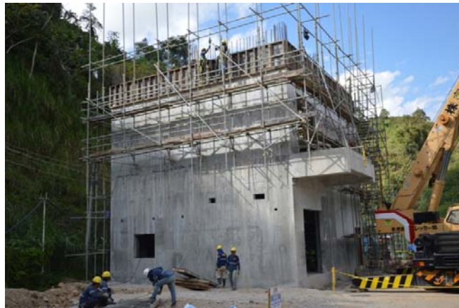
Image10: Process Plant Control Room/Tower
