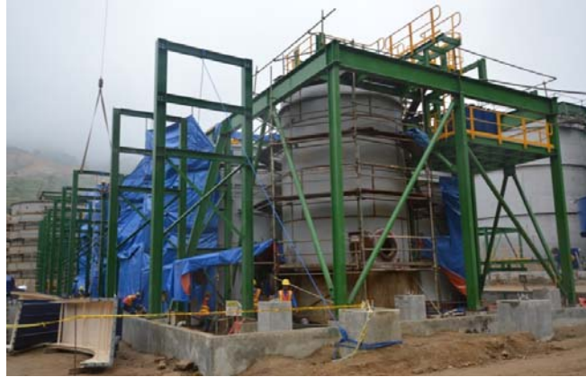
Image 6: CIL tanks and pipe racking
