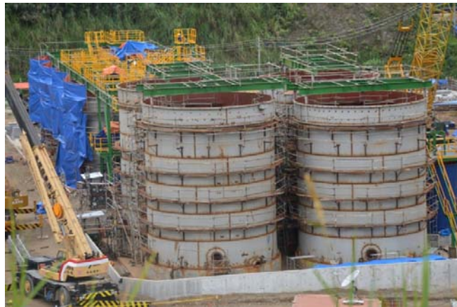
Image 7: ASTER™ and CIL tank area
