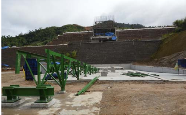
Image 3: Primary crusher area
