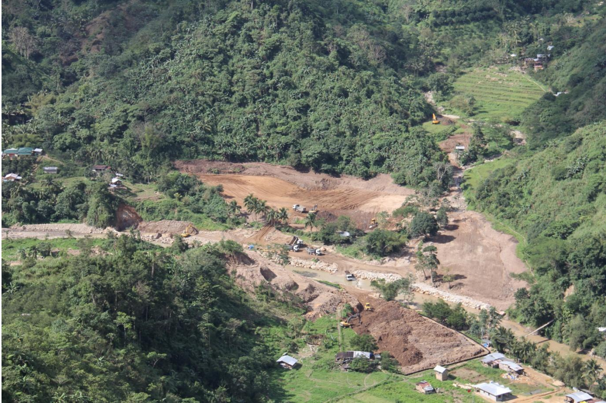
Processing plant site earthworks - looking west from the top of the proposed pit (20 Jan 2012)
