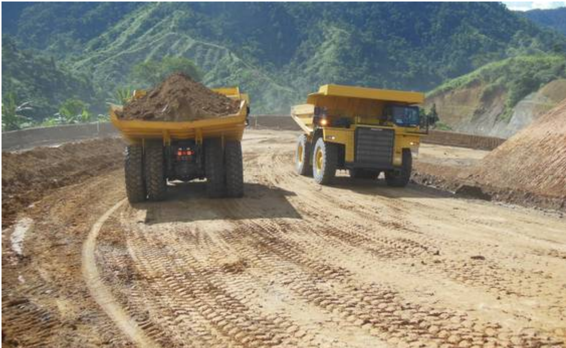
Image 11. Stage 1 pit to ROM Pad Haul Road showing 100 tonne dump trucks passing
