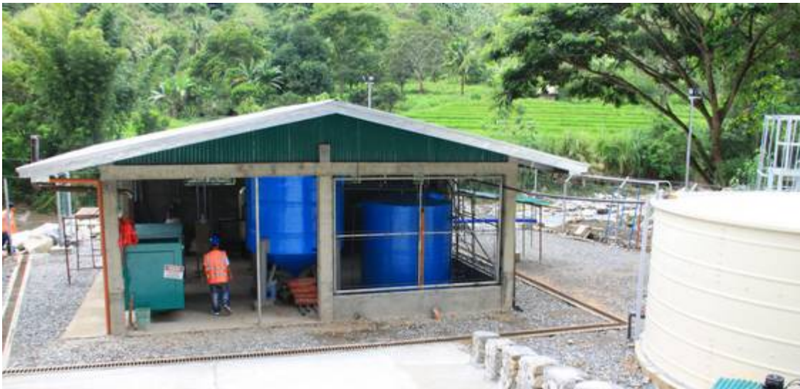
Image 8. Potable Water Processing Plant at the Lintugan River
