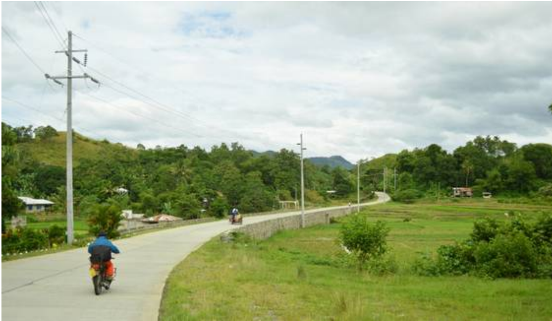
Image 7. Stage One – 69kV powerline Runruno to Maddiangat showing Fibre Optic Cable (top of poles)
