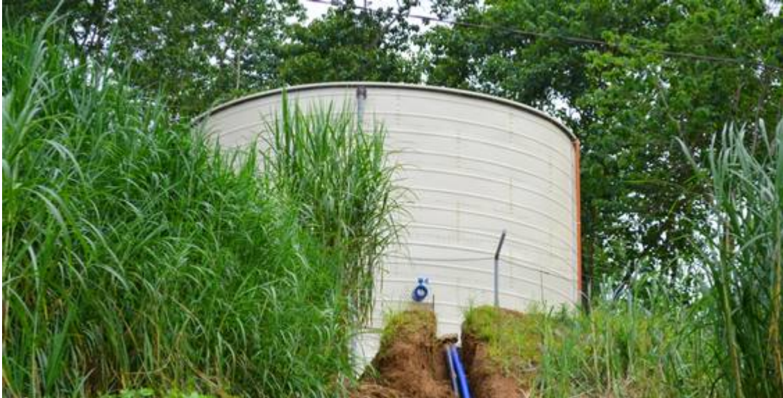
Image 5. Accommodation Area Potable Water Header Tank
