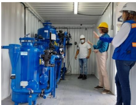
Attention to visit to the plant. Water treatment
