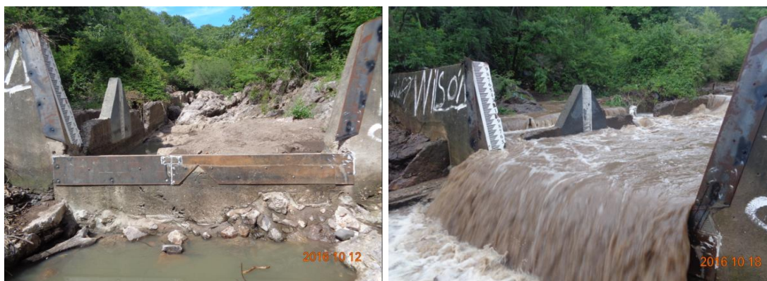
Figure 16-8: La Simona compound weir repair on 12 October 2016 and subsequent flood event on the 18 October 2016
