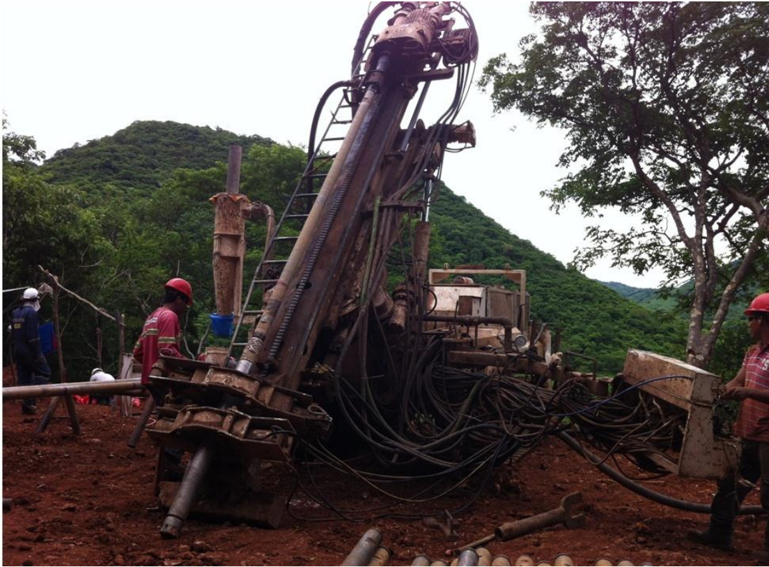
Figure 9-3: Rodio-Swissboring RC Drill Rig being Set Up during the 2012 Drill Program; June 2012
