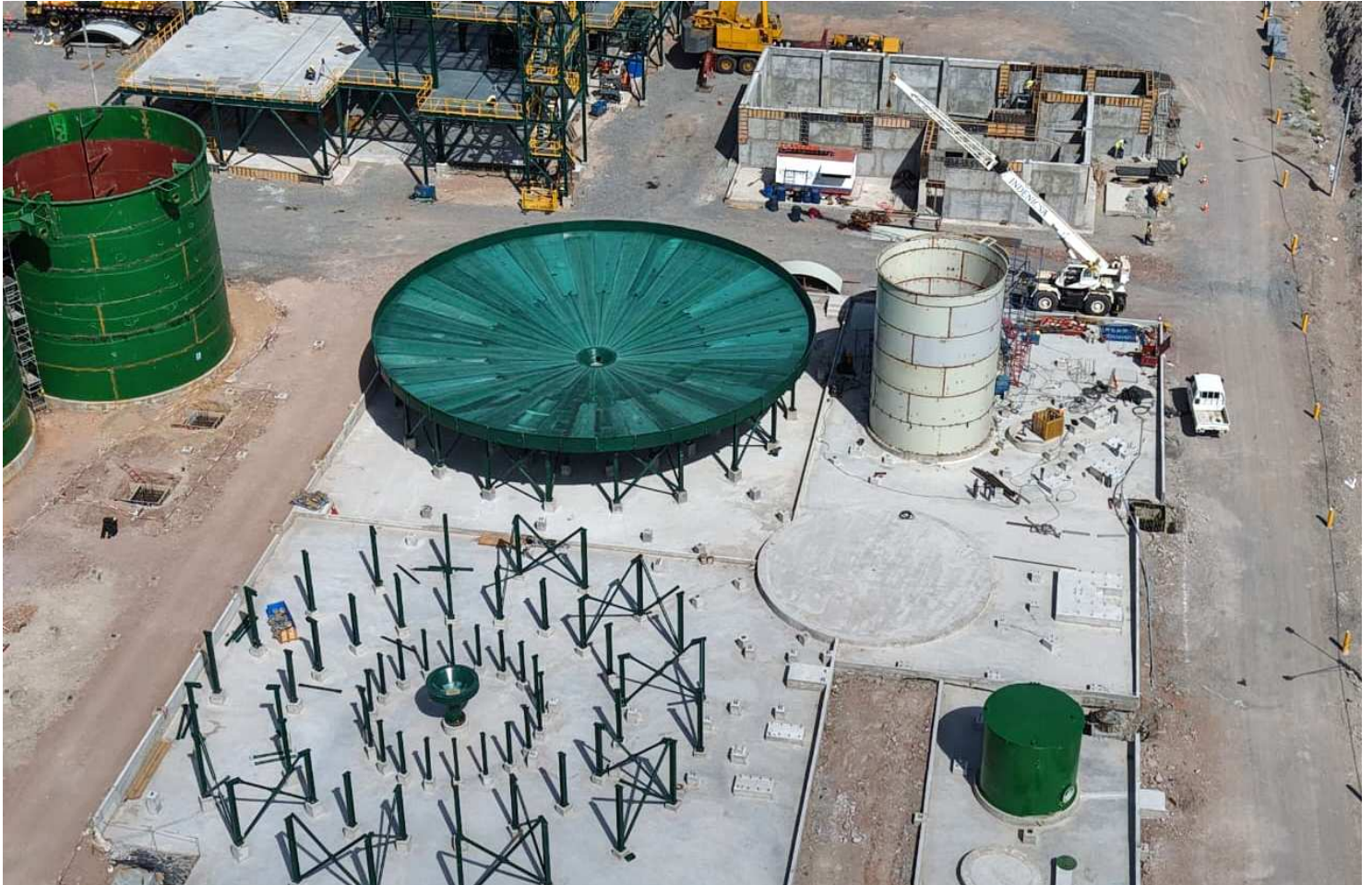
Figure 9: Tailings Thickener Installation & Gold Room
