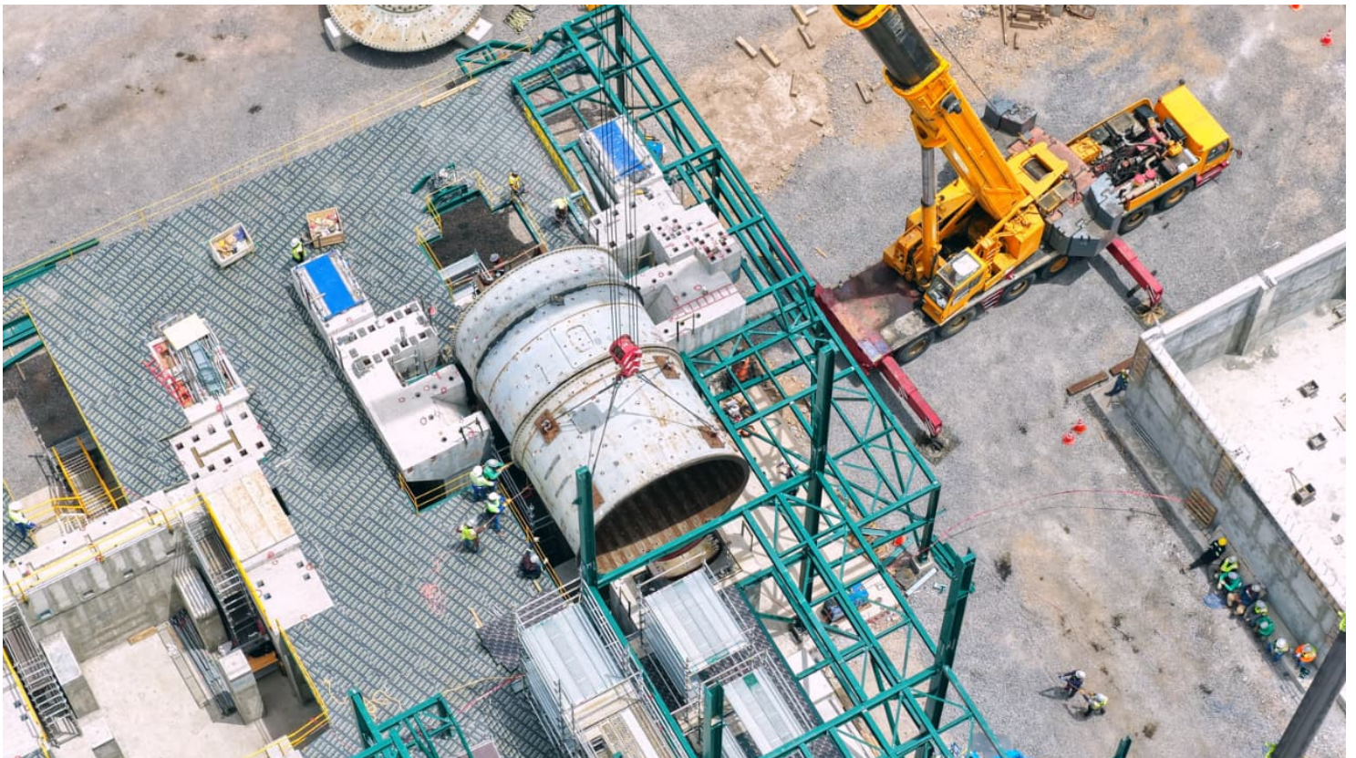
Figure 3: Ball Mill Installation
