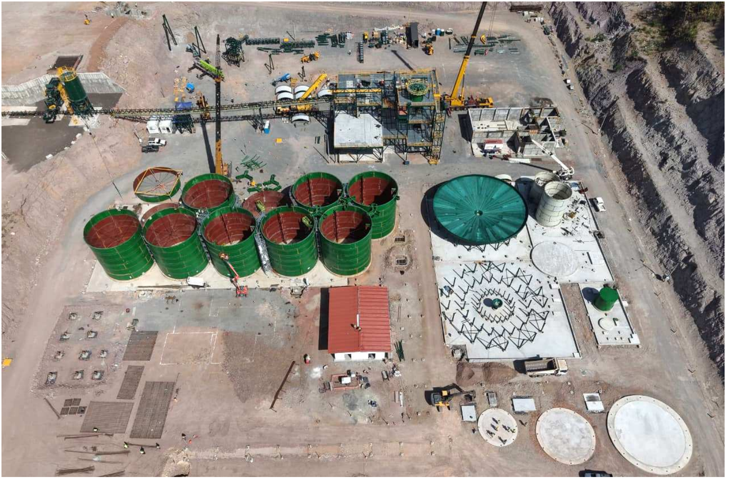
Figure 2: Plant View Close Up
