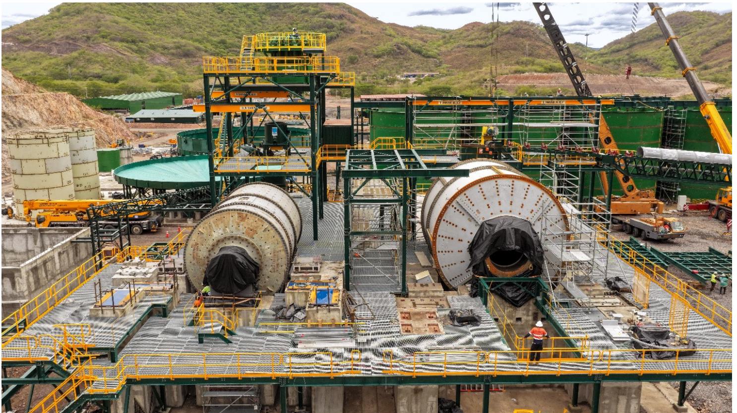
Figure 1: Overall Plant View
